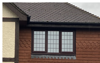
PVC casement windows with a wood-style finish
